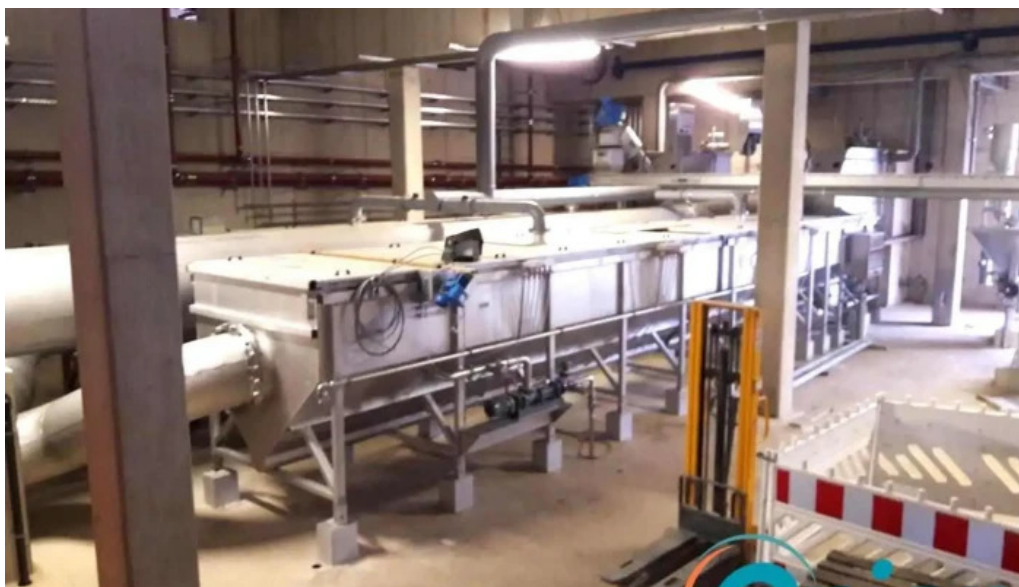
Station d epuration sidest grevenmacher
