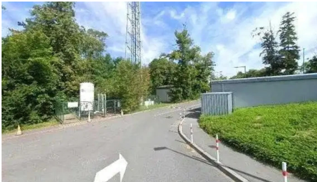
Chargy charging station geigende
