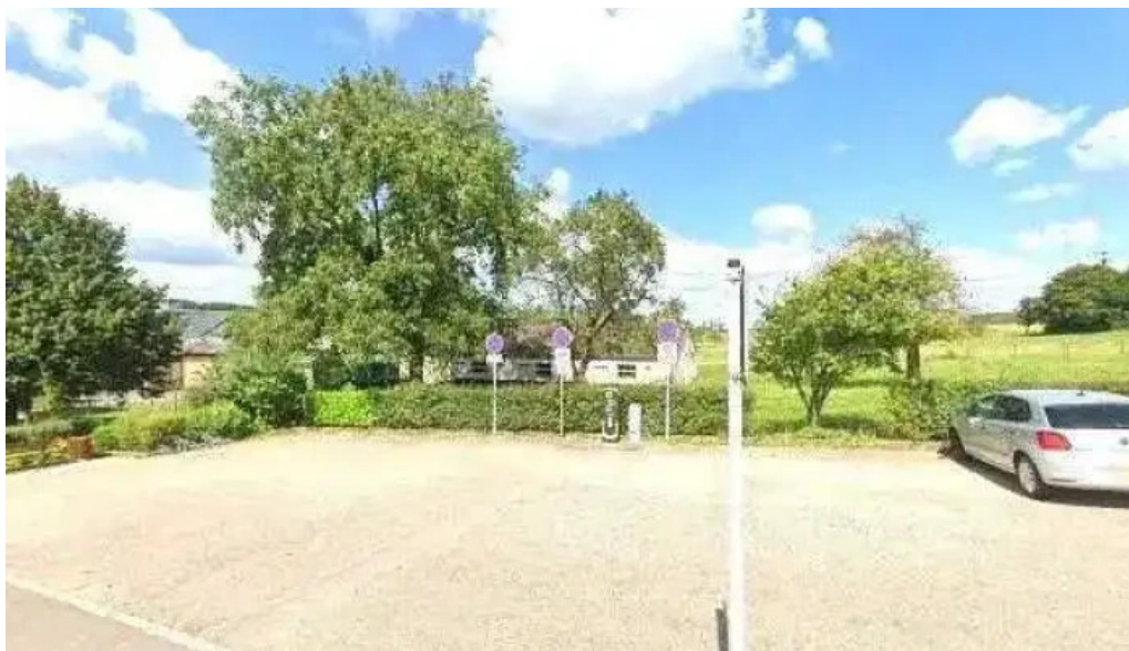
Chargy charging station kommentarene
