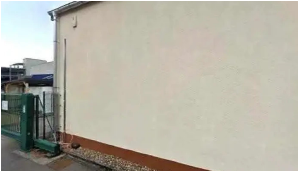
Chargy charging station telefone
