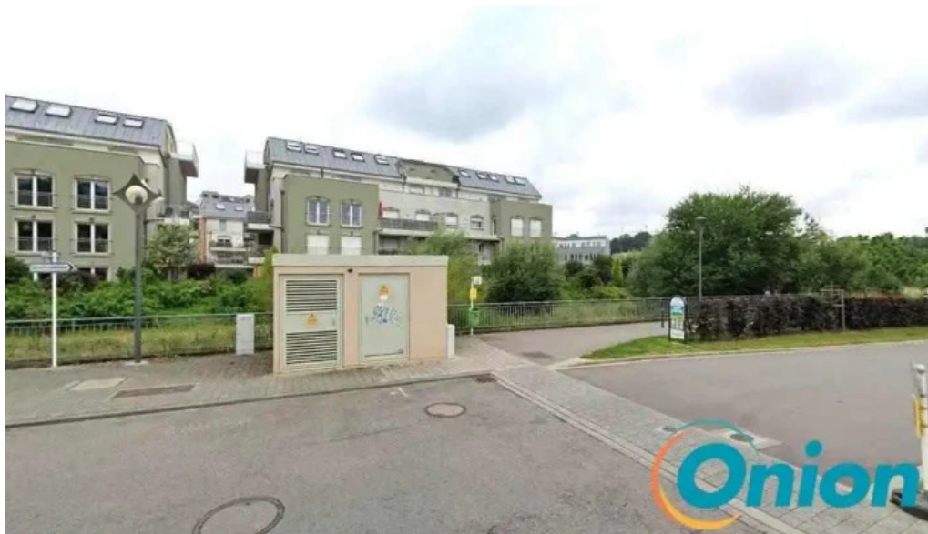
Charge charging station hesperingen
