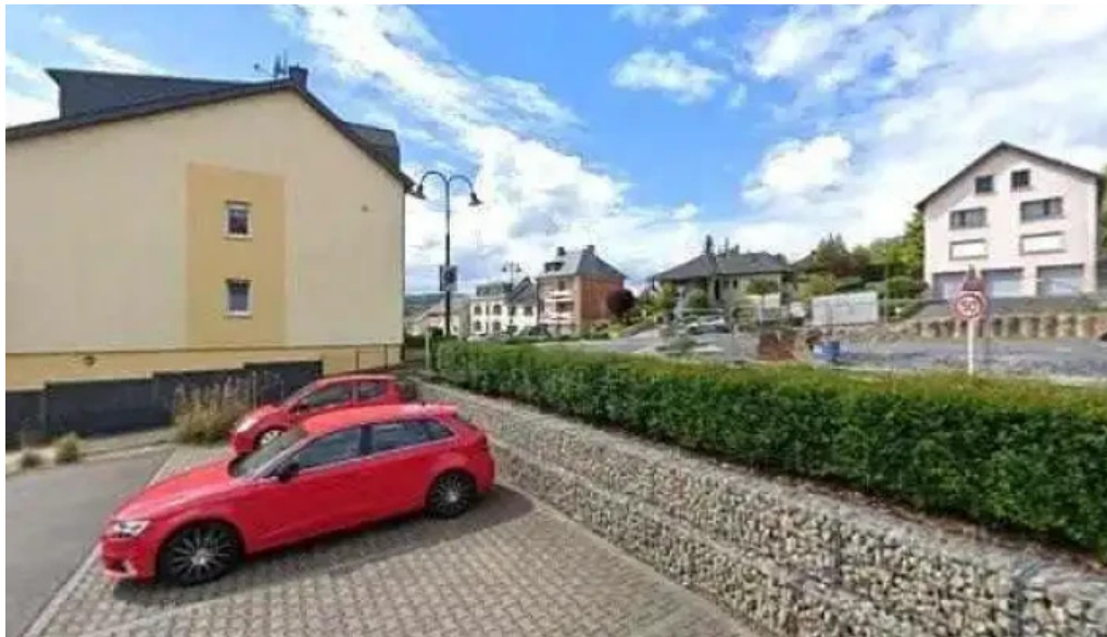
Chargy charging station street view 360deg fotos
