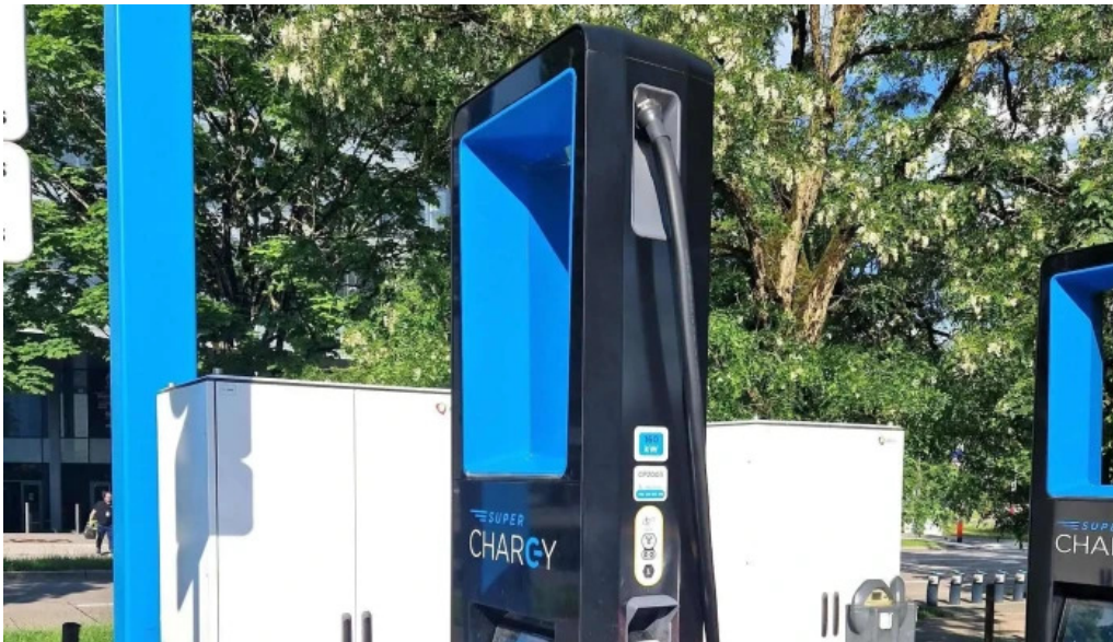
Chargy ladestation luxemburg
