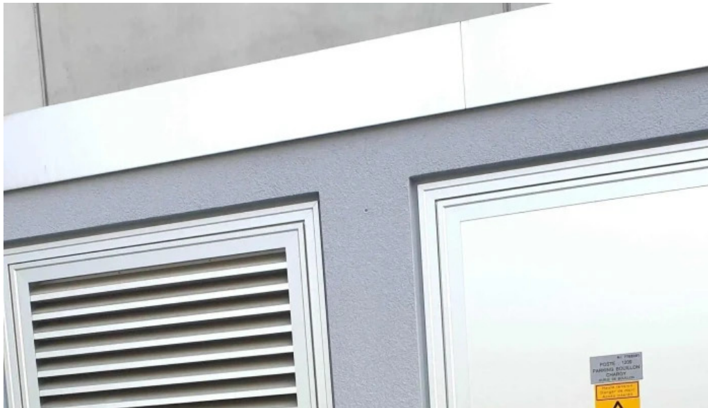
Chargy ladestation luxemburg
