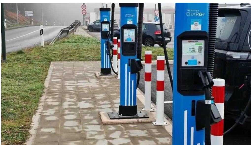
Charge charging station nummere
