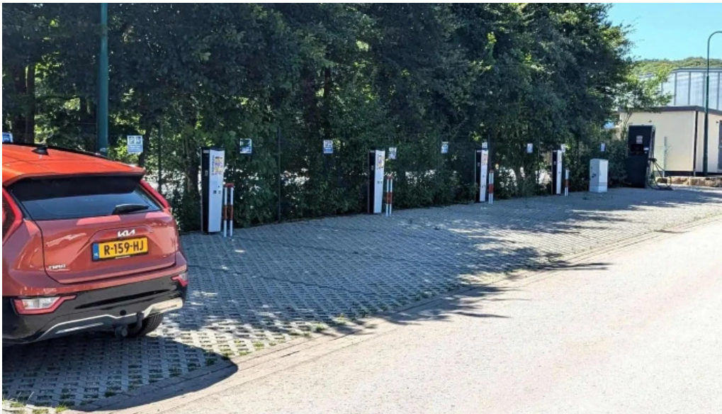
Chargecloud charging station nommern
