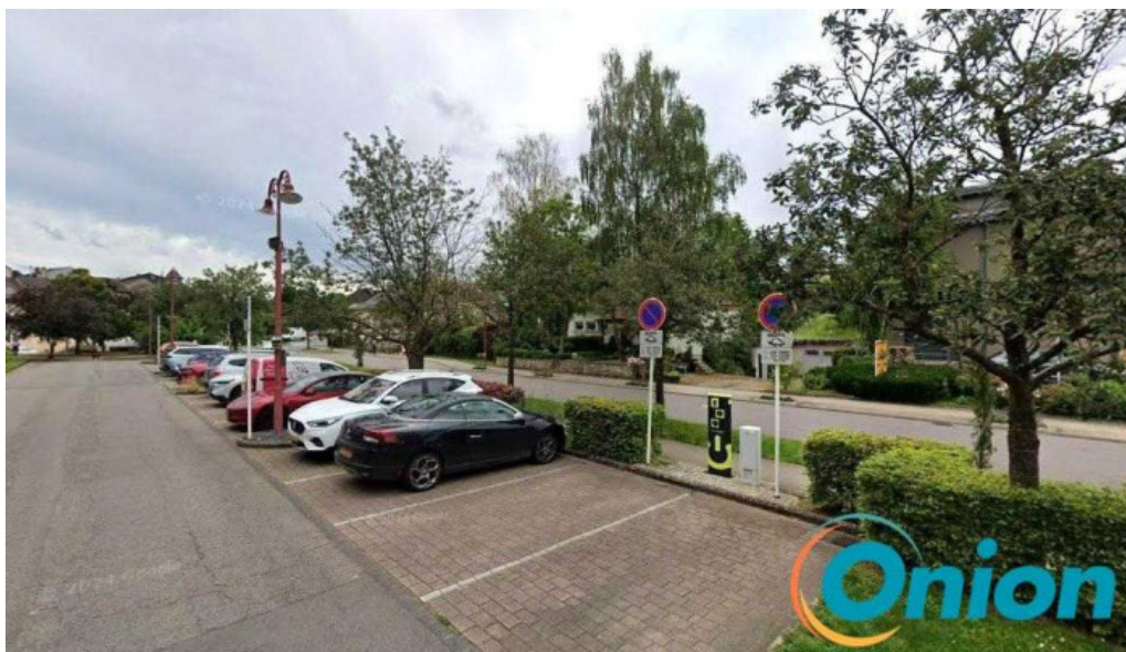
Chargy charging station remich
