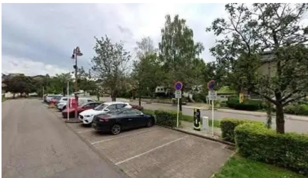
Chargy charging station praisserie
