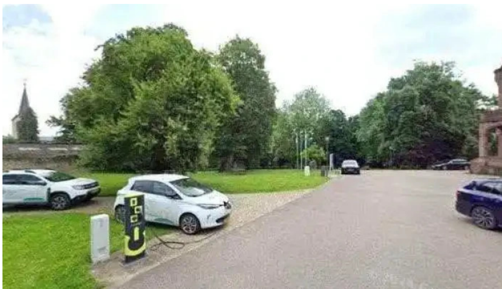
Chargy charging station street view 360deg fotos
