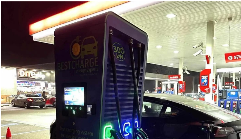
Chargecloud ladestation schengen
