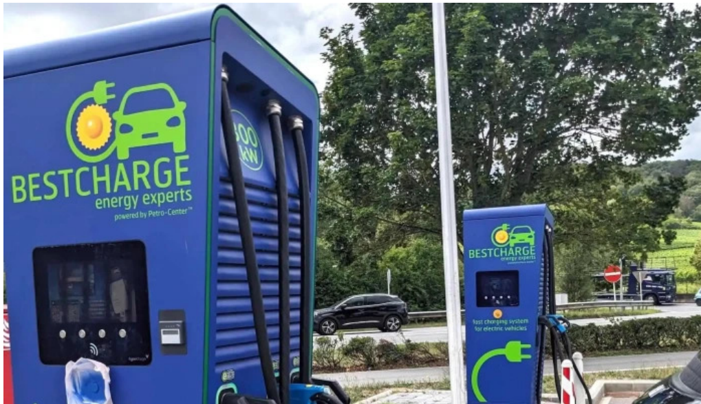
Chargecloud ladestation stonnenplang
