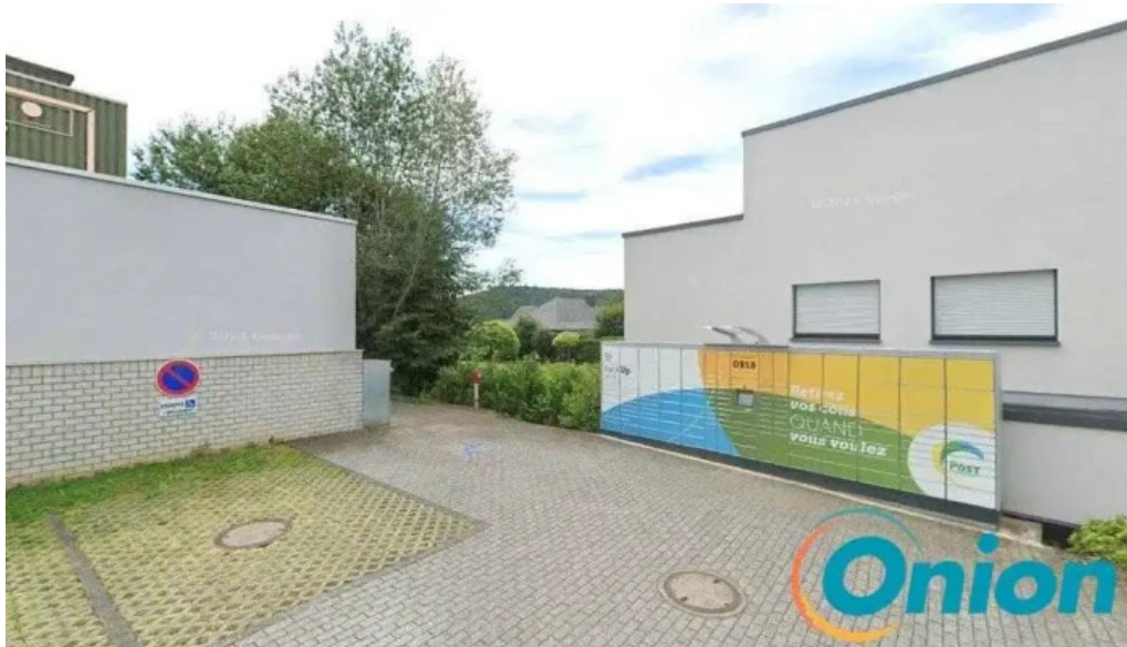
Chargy charging station schieren
